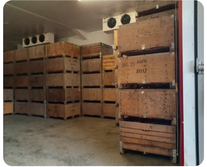
Improving energy efficiency for fruit stores was a high priority for fruit growers in the Growing Green programme
